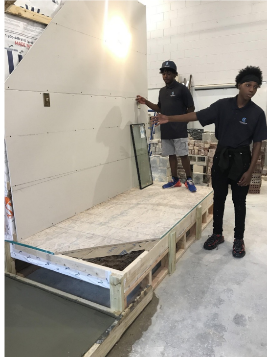
Building a Passive House Wall Assembly Mockup for use at Carver House
